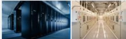
DATA CENTER DESIGN & INSTALLATION
